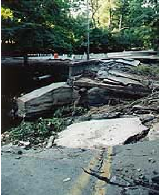
(Dam failure following Hurricane Floyd, Fall 1999. Source: NC Division of Pollution Prevention and Environmental Assistance)
