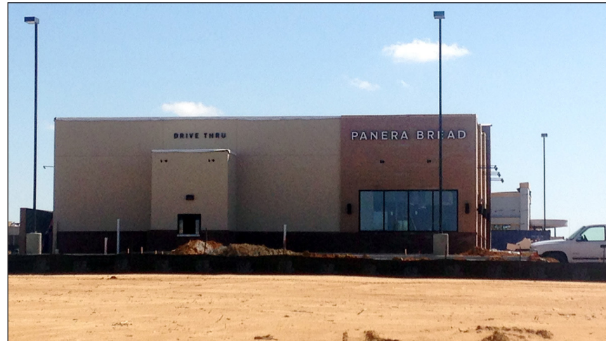
Construction is well underway on the Panera Bread restaurant slated to open in the spring at the intersection of U.S. 70 and Jones Sausage Road.
